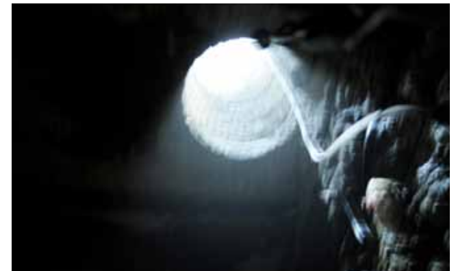
Trout Brook Storm Sewer, 2010
